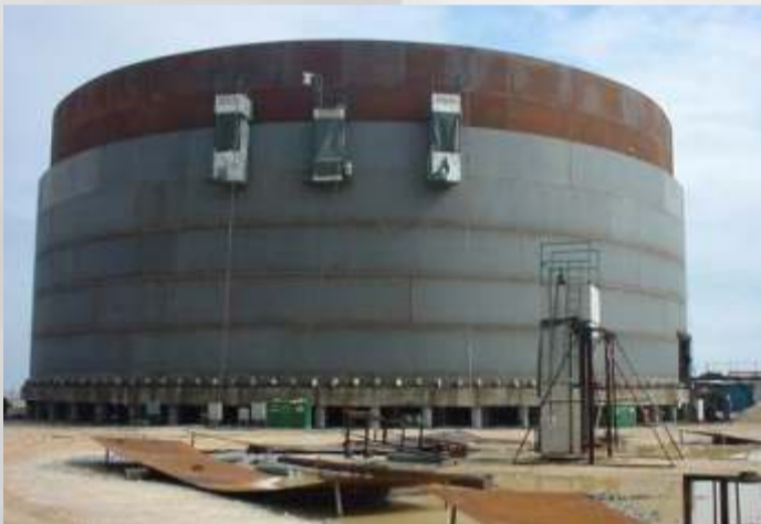
Double shell LPG Tank
